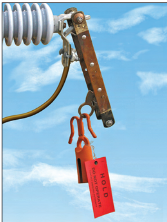
R-TD installed on a disconnect switch
